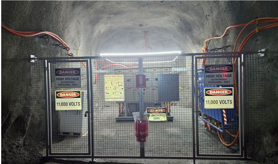
Figure 14 - Underground electrical sub-station
