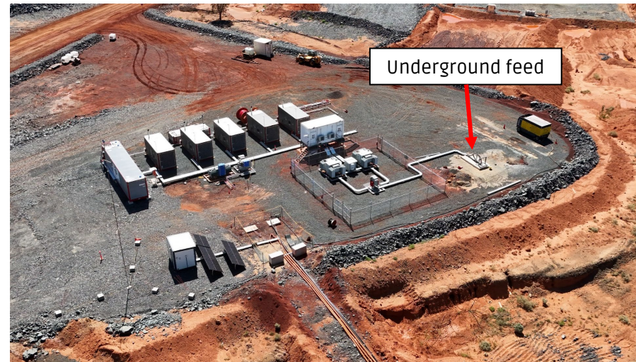
Figure 11 - Expandable 2 MW Power station and showing underground cable feed
