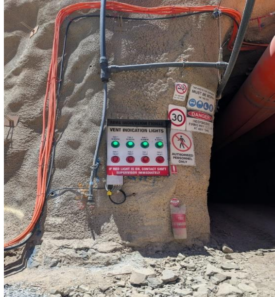
Primary vent fan indicators
